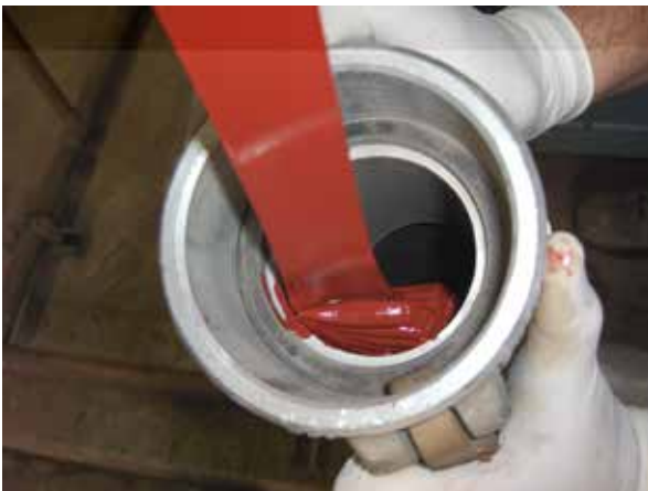
The epoxy is blown through the pipe system to create an even coat, which will cure (aka: dry) and create a protective liner.
